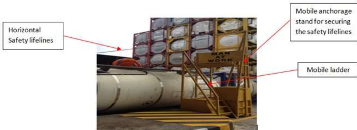
Figure 2: Worker working at the top of the tank with his safety harness anchored to the safety lifeline.
