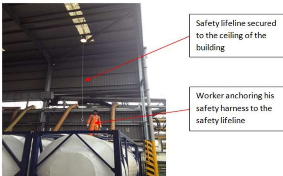
Figure 3: Lifelines secured to the ceiling of the building when work activities are carried indoor.
